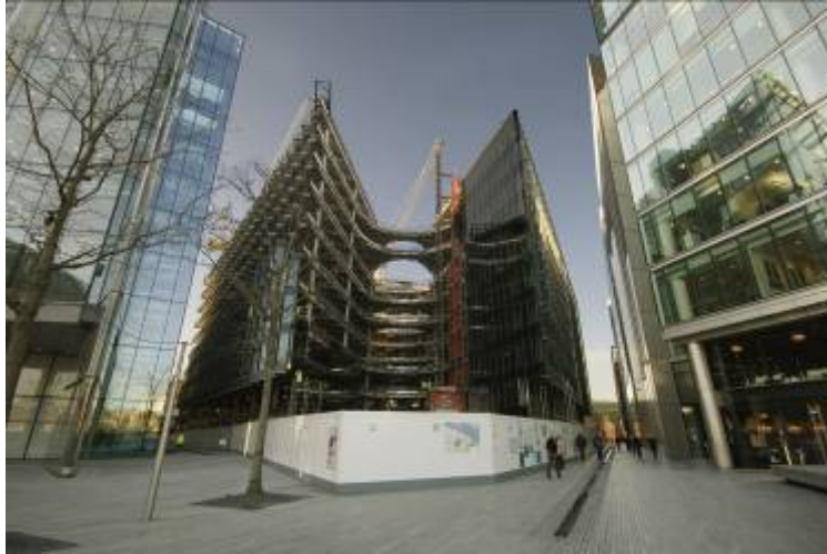
Promat UK has supplied fire protection and thermal upgrading solutions to the 7 More London Riverside project.
