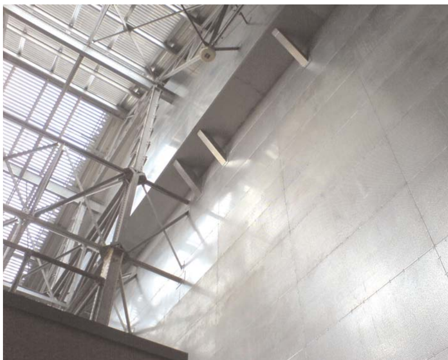
The tallest ever DURASTEEL® firewall in the UK, inside the DIMCO building.
