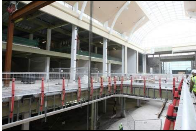
CAPTION: Over 150,000 m 2 of Promat PROMATECT ® -250 non-combustible board and Promat TD Board ® inert mineral fibre board have been used to protect the Centre's structural steel elements
